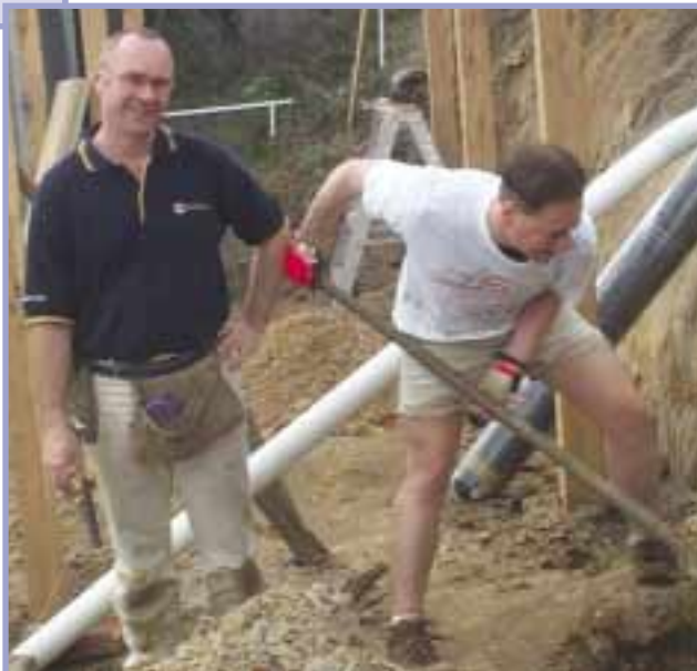
Greg with builder Russell Joseph assisting volunteers at the Mt Martha bowls club with the construction of ramps for disabled and wheelchair-bound bowlers
