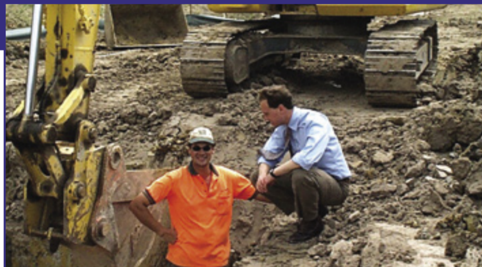
Greg inspecting progress on the newly completed slipway on the Western Port Hwy near Hastings and Tyabb, to which the Commonwealth contributed $300,000.
